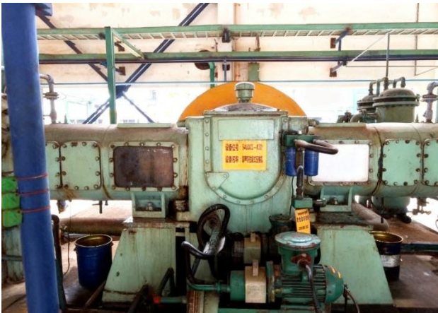
A picture of the Compressor #1
